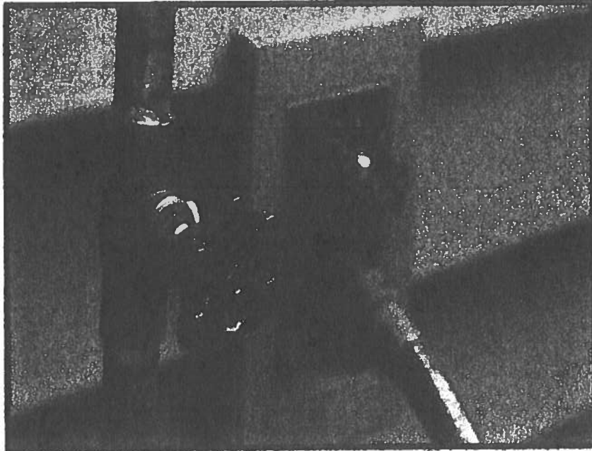
Figure 30: Example of Water Shut-Off Valve
